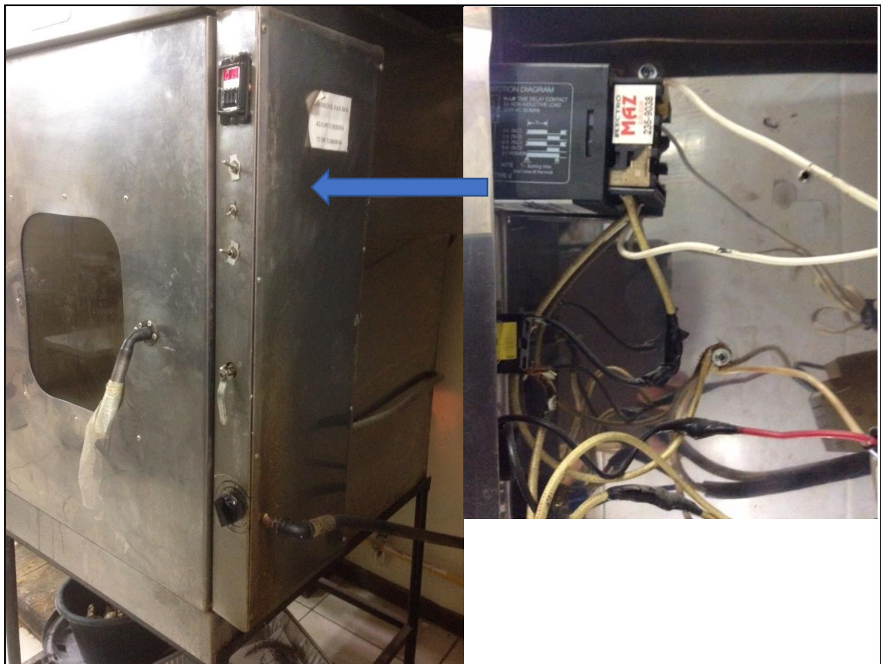
Figure 26: The Oven controls cabinet before the upgrade to the automatic system
