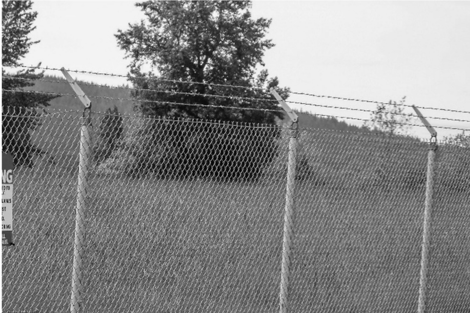
Figure 13 Perimeter Fence Barbed Wire Top Cap Facing the Wrong Direction – Facing Away from the Threat (Photo by Ernie Hayden)
