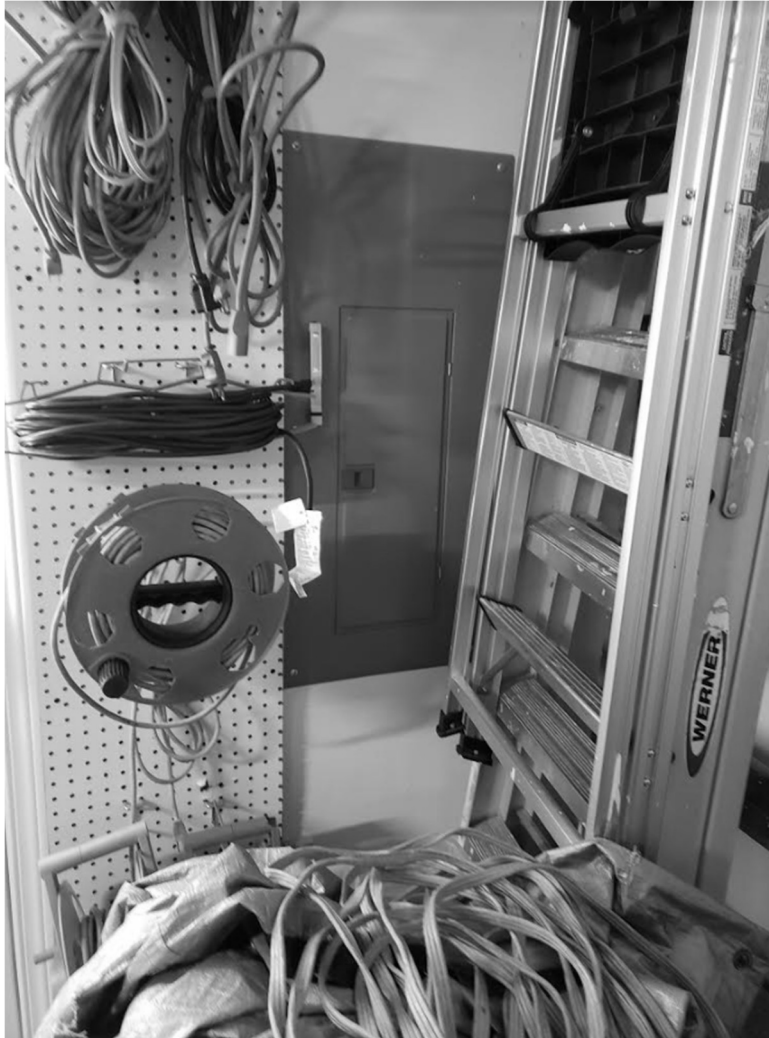
Figure 15 Blocked Circuit Breaker Panel (Photo by Ernie Hayden)
