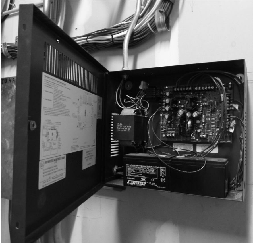
Figure 8 Open/Unlocked Control Cabinets
