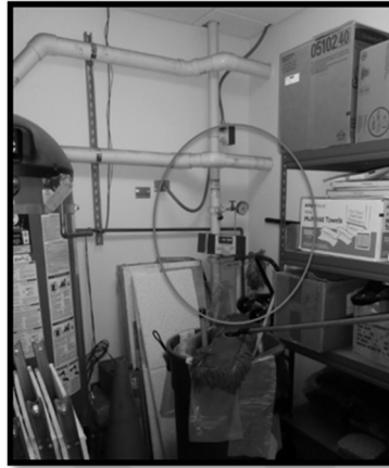
Figure 21 Sprinkler Riser is Blocked in a Storeroom
