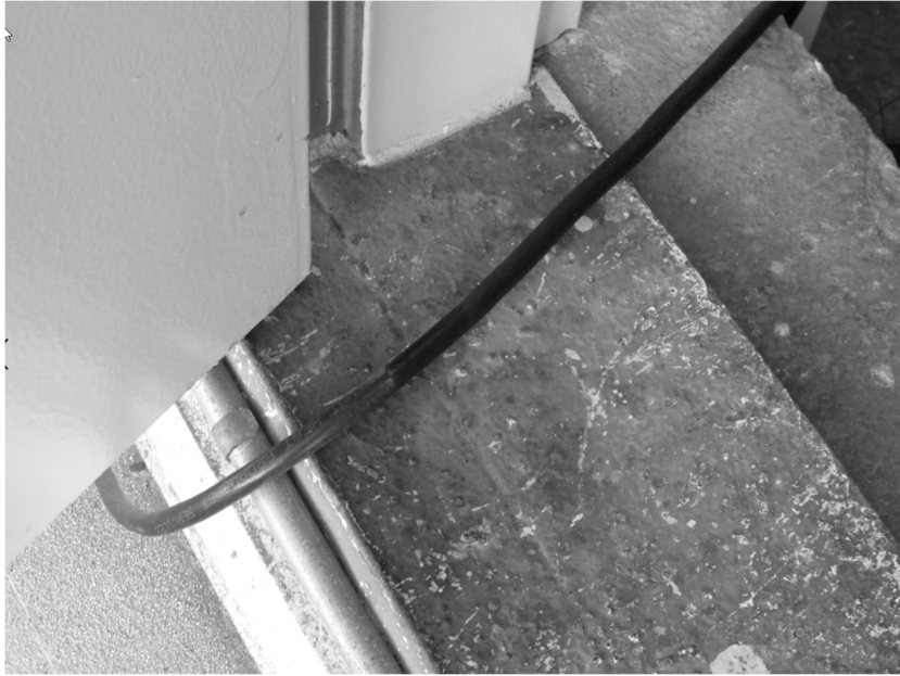
Figure 12 Cable Running Across Door Threshold (Photo by Ernie Hayden)
