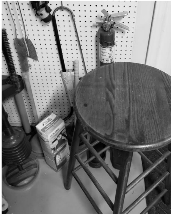
Figure 14 Blocked Fire Extinguisher (Photo by Ernie Hayden)
